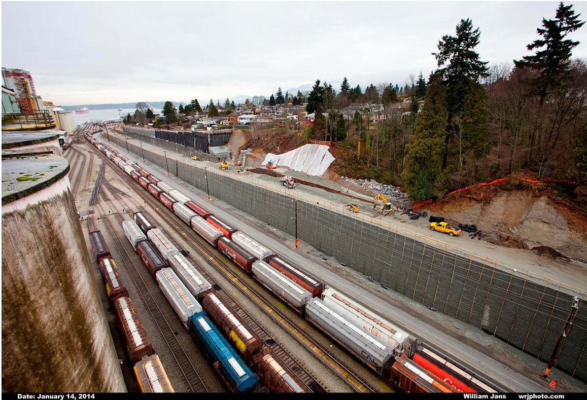
Top of grain terminal, looking west, showing the new Low Level Road alignment along the lower wall and the Spirit Trail on the upper wall.
