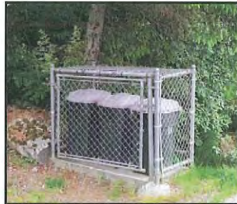
Chain link enclosure - this one would be more secure without the gaps between the panels and the posts. Strengths: Built on concrete slab, anchored to ground. Weaknesses: Needs roof to shed snow/water. Lots of places for bear to grab and pull. Cans visible to bears.
