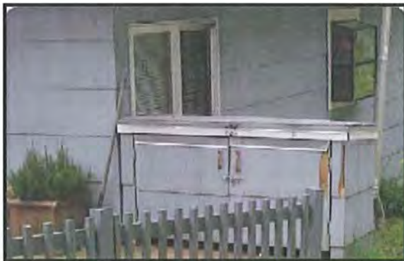
Wood enclosure. Strengths: Secured to ground, sturdy latch, metal flashing on roof seam. Weaknesses: Matching siding too flimsy.
